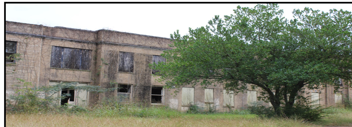
Once a building that provided needed health, the T&P Hospital now shelters homeless, vagrants, and the occasional ghost.
